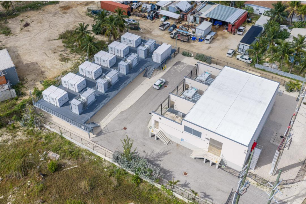
Battery Energy Storage Systems (BESS) installed and operational
